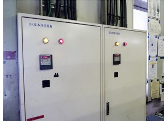
A power meter is installed at the FOL-3015AJ's power source to monitor electricity usage in real time
