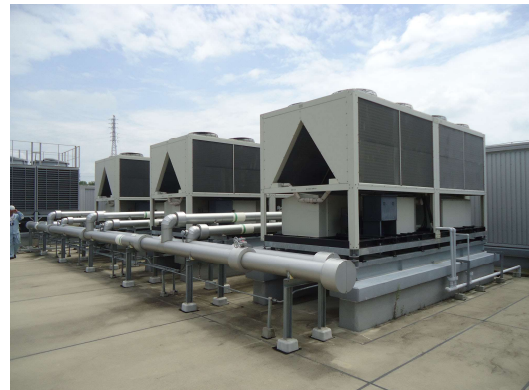
Water thermal storage system air conditioning chillers (Toki Works)
