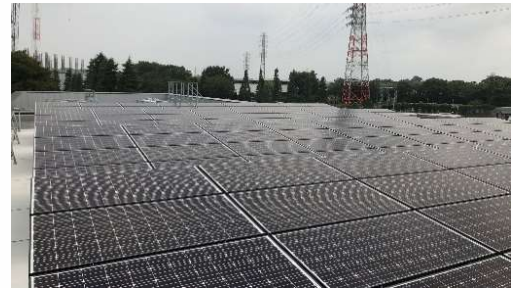
Solar panels installed on the rooftop
