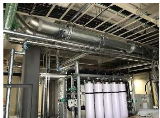
Well water filter
