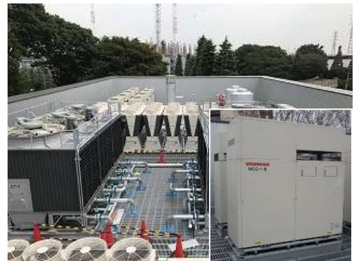
Micro cogeneration units
