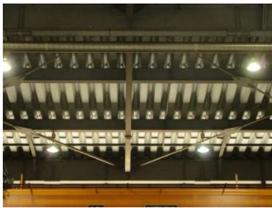
Original mercury lamps
