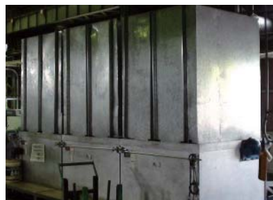
Promoted heat insulation for the tempering furnace (Miki Plant)
