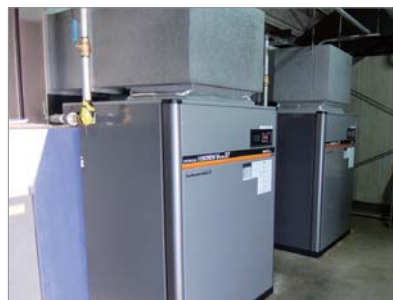
Energy saving compressors (Ono Plant)
