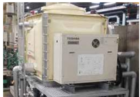
Waste heat use (Ono Plant)
