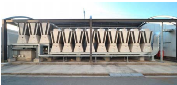
The heat pump chiller at the Ono Plant
