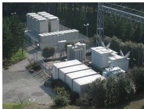
Fujinomiya Works: NAS battery
