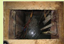
The activated bio tank
