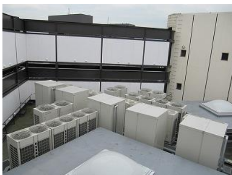
Isehara Works: “eco ice” in the headquarters building
