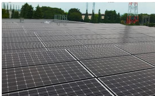
Solar panels on the Disaster Management Energy Center rooftop (Isehara Works)
